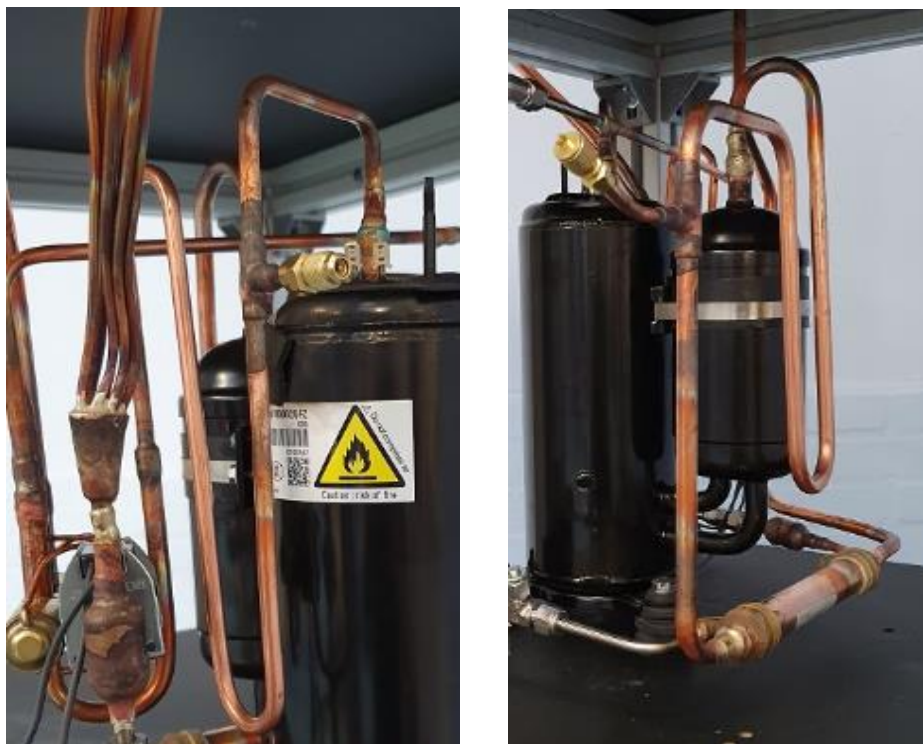
Figure 4: Additional length for flexibility in the tubing. Left: Discharge tubing. Right: Suction tubing.
